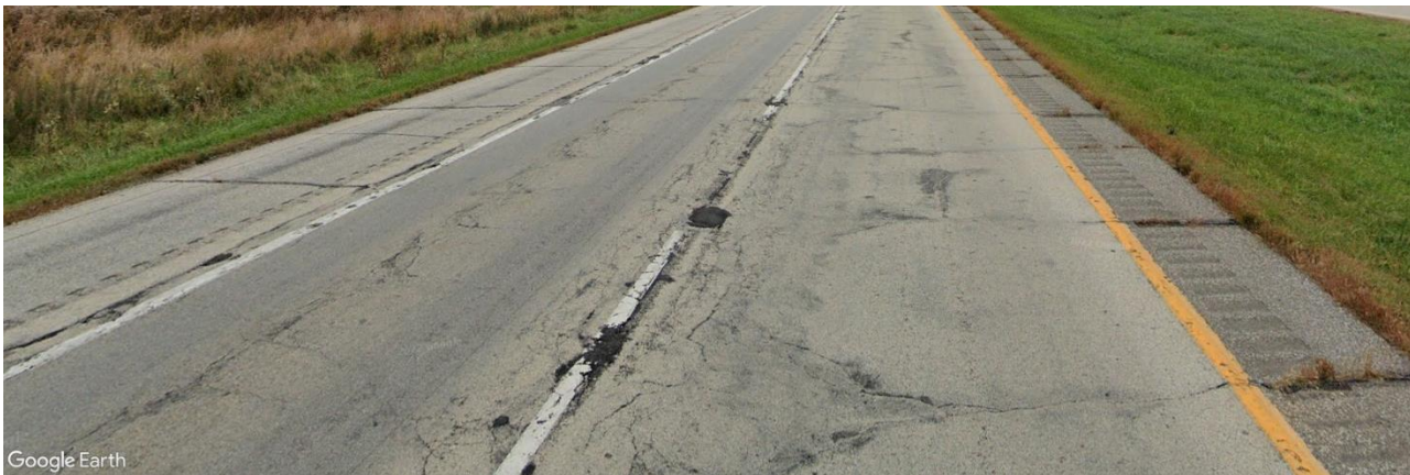
Figure 5 – US 30 Pavement (Oct 2022)
